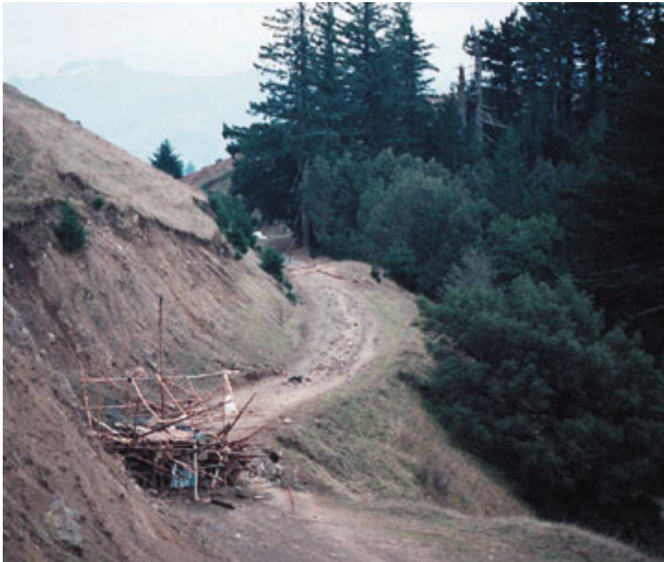
Clearcut in progress in a steep slope of Rainbow Ridge (2002) The denuded hills, once they trees that hold them together are cut (along with all other vegetation) erode easily with the first rains, ending up as sediment in the river. Courtesy of Trees Foundation.
